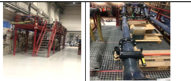
Picture: Water pipe separator in laboratory
