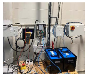
PV controllers for testing
