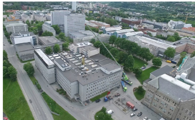
TOWER: On 1 July 2016 a tower was lifted through the roof of the thermal engineering laboratories (Varmeteknisk), which measures from floor to top about 20 meters. It was raised in two parts; first an internal staircase and then an outside tower with stairs. The tower provides an extension of the multi-phase flow laboratory. Photo: Jørgen Hjelmøy, Ufo2 AS
