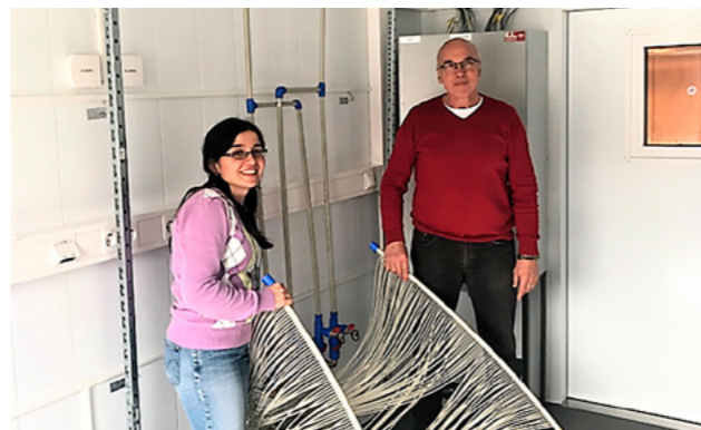
ON THE INSIDE: Natasa and Eberhard Schmidt, from the company Wasserkabel, are placing and testing water capillary mats that can be used for heating, cooling, and dehumidification.
