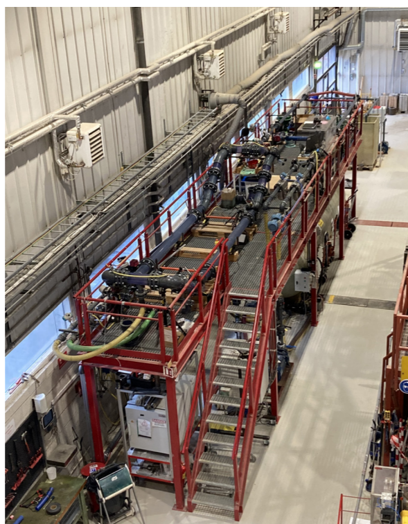
Figure 4a) Photo of the experimental facilities, depicting the separator, control station and flow meters on the top floor and pumps, storage tank on the ground floor.
